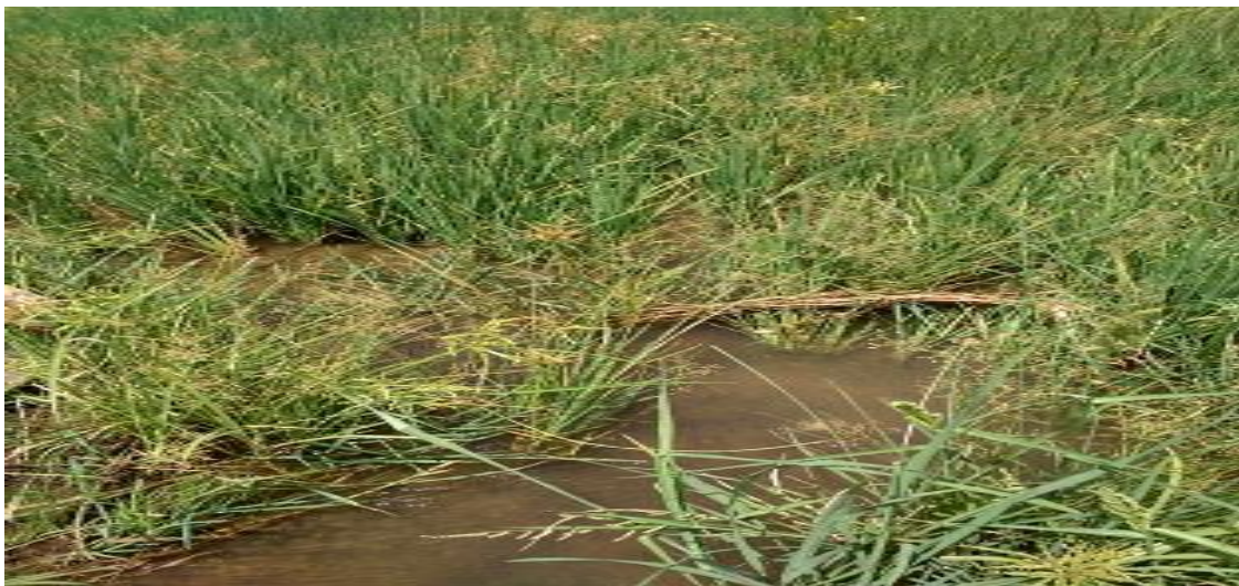
Plate 4.1: Condition of Field Drains of Bontanga Irrigation Scheme
